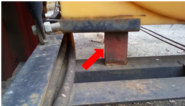
Fig. 11. Installed left mounting pad with support
